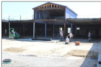
Exterior architectural rendering – Construction is being working on the courtyard at the new Rock Island Village elevated living facility. The development has transformed the former Cannon International facility on E. Eighth Street in St. Louis.
