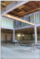
A look at the atrium – Construction is progressing on the new Rock Island Village. There is what will be an atrium area that will also include a living area and lounge.
